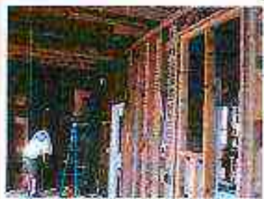
The Inn's stairs first to be taken down in the month before restoration can begin.
